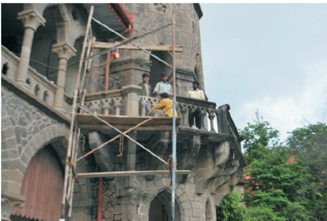
Conservation Of The Central Balcony At The Deccan College By Basalt Stone Workers
